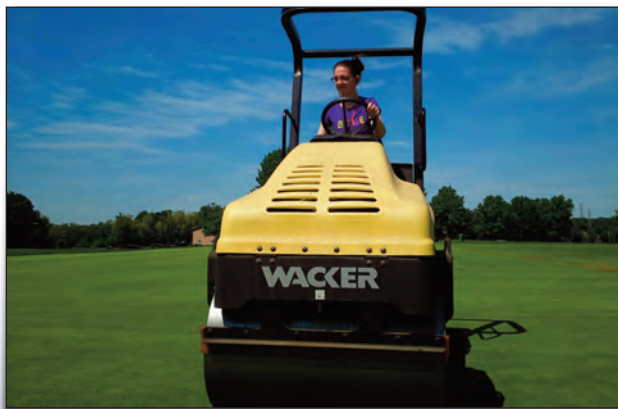
Traffic was applied to the plots with a 1.7 metric ton, smooth-drum, vibratory asphalt roller with four passes, five days a week from June through October.
